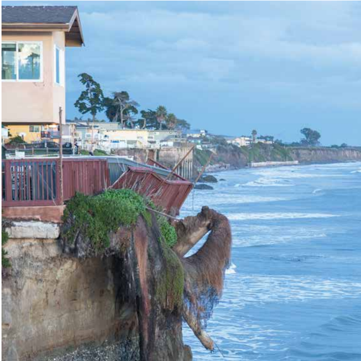
SLAMMED, JAMMED, AND CRAMMED: Mother Nature shows she doesn't care a lick about UCSB housing shortages or Isla Vista landlord profit margins as erosion continues to do what erosion will continue to do.
